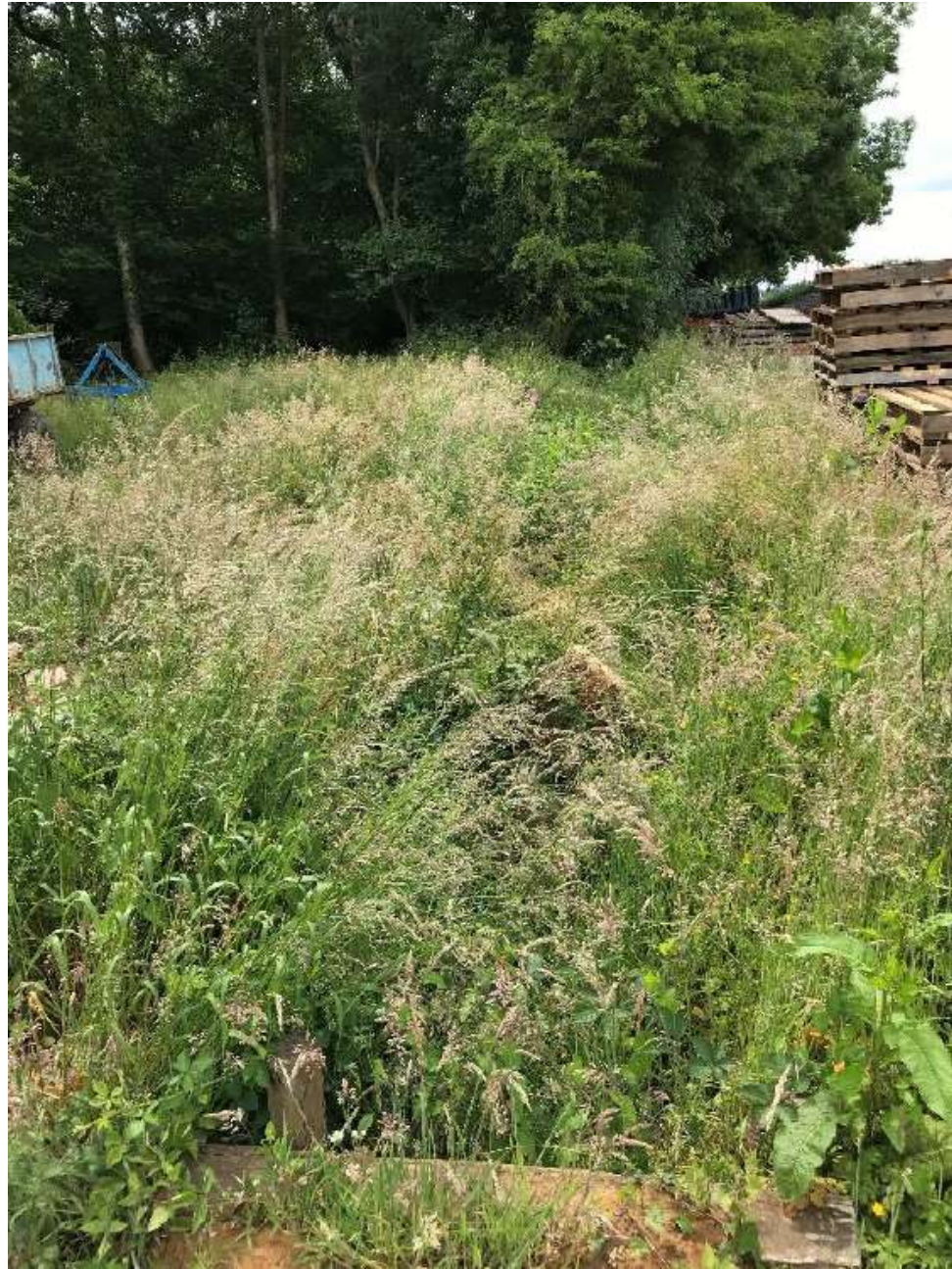
View of existing drainage ditch between existing farm yard and woodland (looking south)
